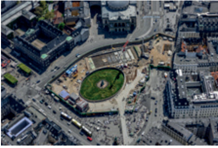
An aerial photo of the construction works for the new Metro station in Copenhagen near the Magasin du Nord. The store is at the top right of the photo
